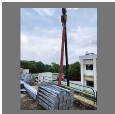
Solar Panel Mounting Structure
