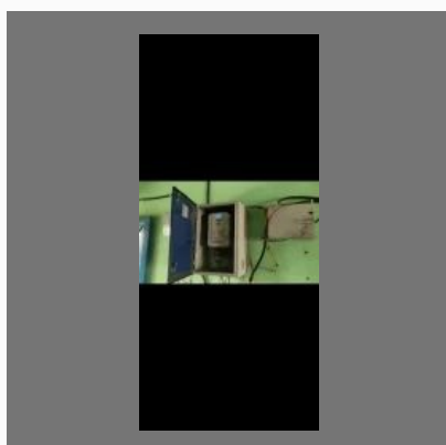
Solar Vfd Drive
