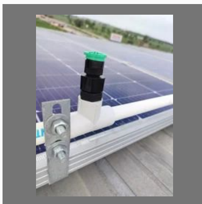
11 Zone Solar Panel Cleaning System
