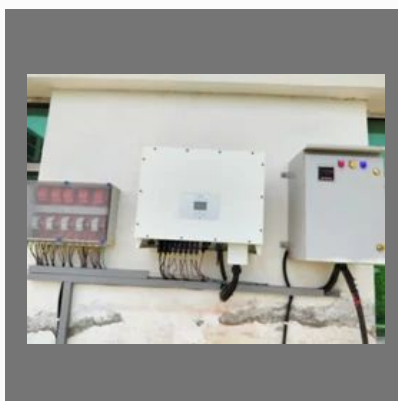
Solar Panel System
